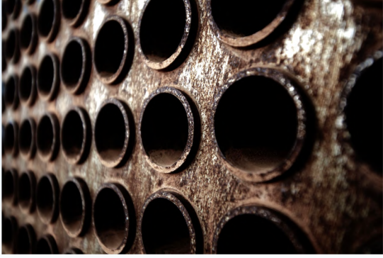
Corroded heat exchanger from condenser
